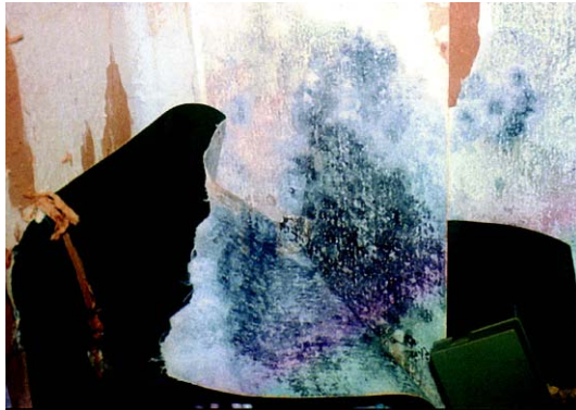
Photo 5: Mold growth behind wallpaper
