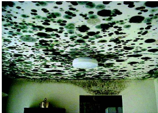
Photo 2: Extensive mold contamination of ceiling and walls
