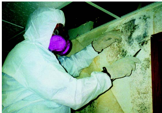
Photo 7: Remediation worker with limited PPE
